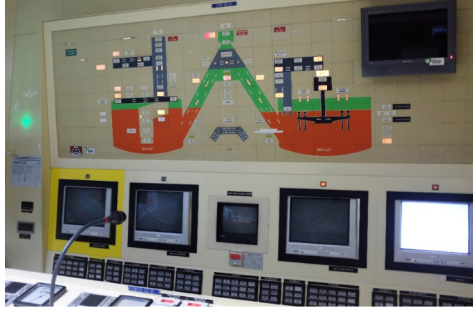
Figure 6. Phénix Control Room
